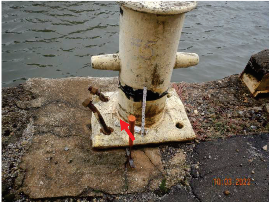
Photo 23: Failed bollard along the South Apron
