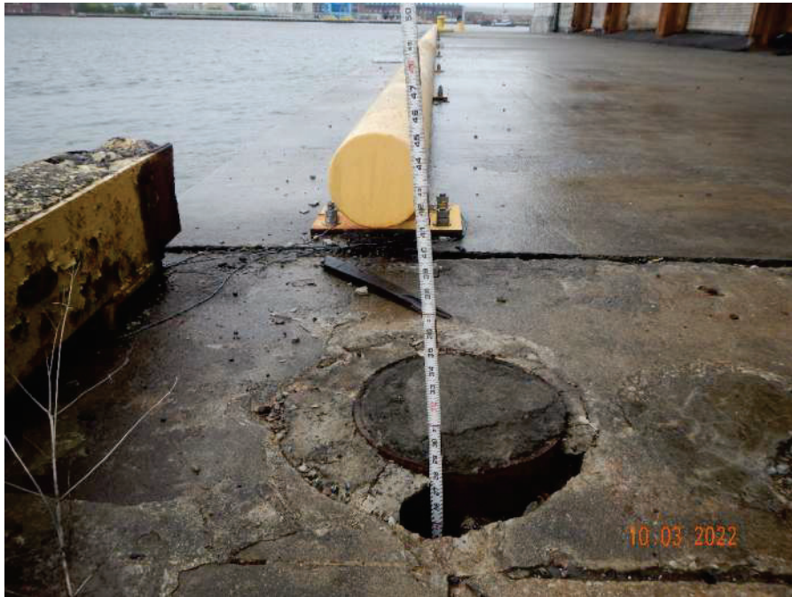
Photo 13: Isolated areas of spalling at Aux. steel pipe pile
