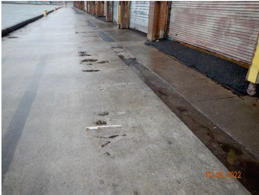
Photo 11: Typical shallow spalls in top of deck
