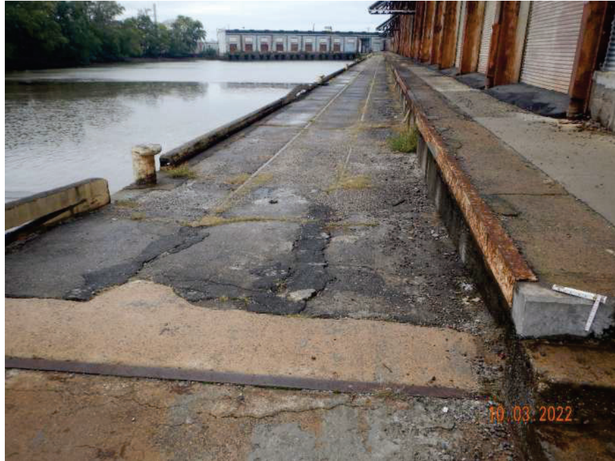
Photo 19: Typical failed asphalt along South Apron
