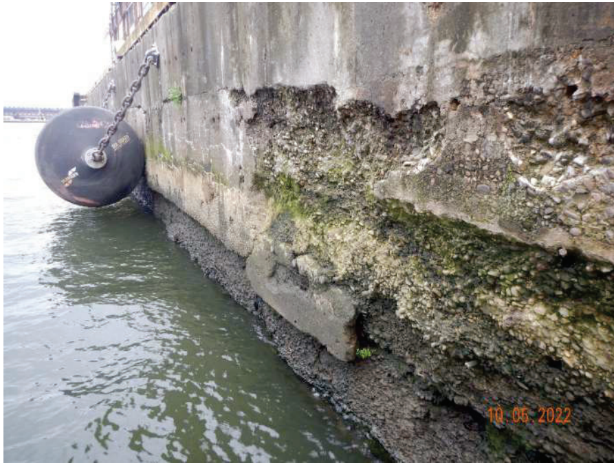
Photo 25: Typical spalling along deck fascia
