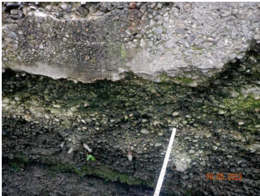
Photo 26: Typical spalling along deck fascia
