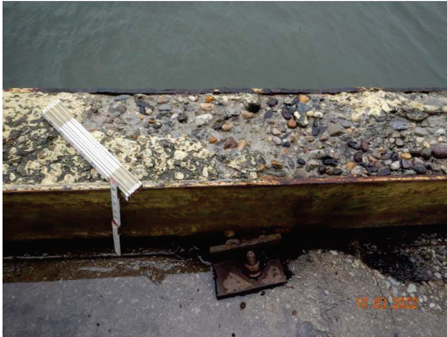
Photo 17: Typical failed curb connection (North Apron shown)
