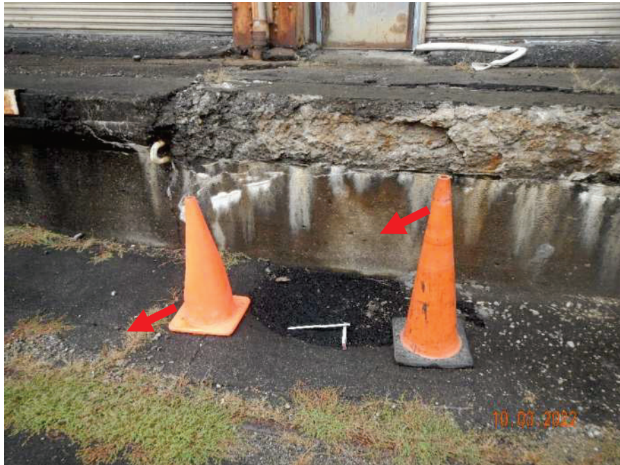
Photo 20: Recently patched sinkhole on South Apron
