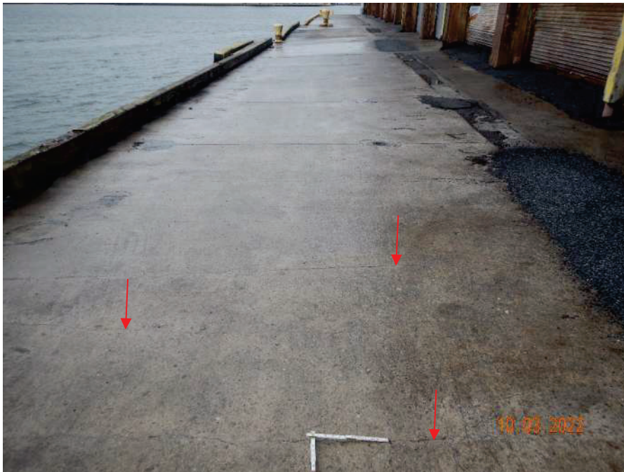
Photo 9: Typical transverse cracking in top of deck (North Apron shown)
