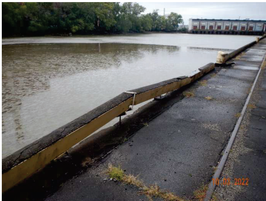
Photo 18: Typical failed curb (South Apron shown)
