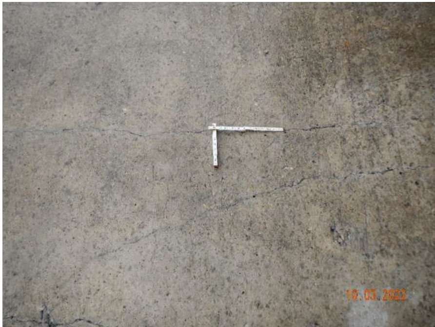
Photo 10: Typical transverse cracking in top of deck (North Apron shown)
