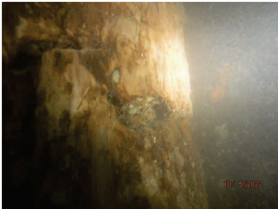
Photo 30: Typical broken timber pile
