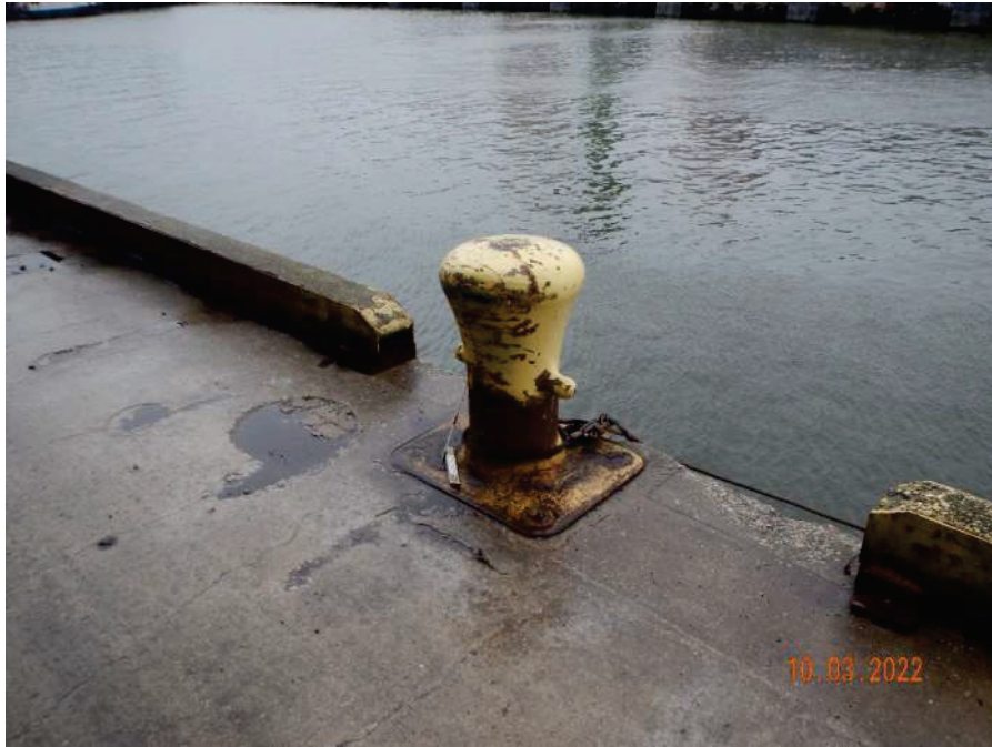
Photo 21: Typical bollard with minor to moderate corrosion
